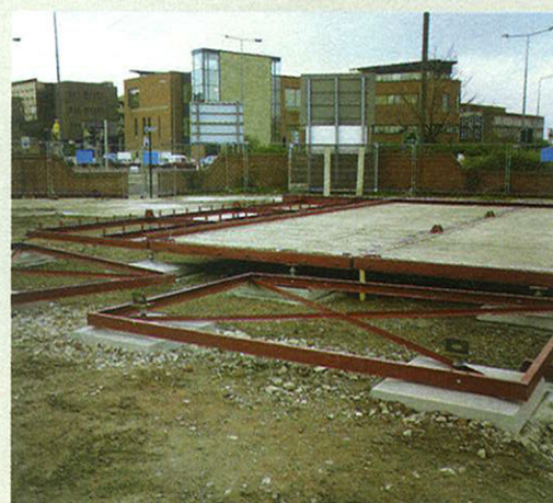
The foundations being positioned on site are a series of precast concrete padstones which sit on the ground. The floor is made from steel-framed cassettes bolted together and filled with ballast to resist wind uplift.
